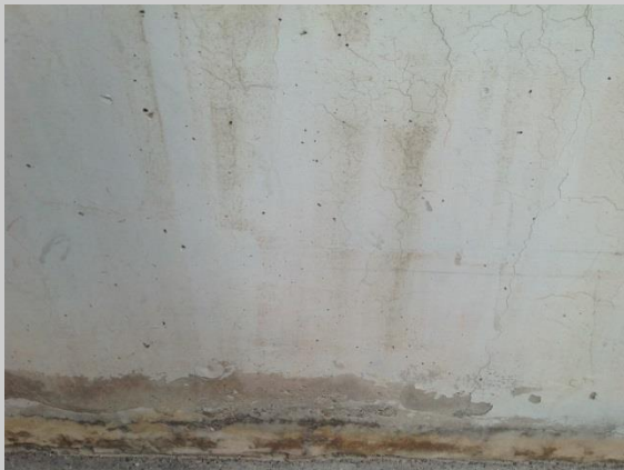
Destruction by salt spreading
