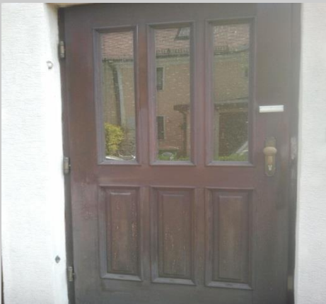
weathering of a wooden door
